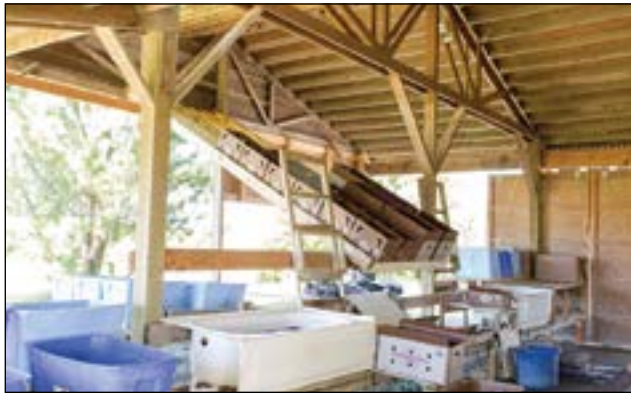
An open-air packing shed must be kept clean and regularly monitored for wildlife, pooling water or other contamination risks.
